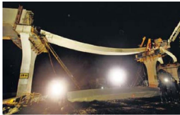
Fig.2 Elevated section of the tracks under construction came crashing down in Delhi Metro
