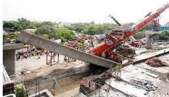
Fig. 3 Concrete beam collapses at monorail site in Mysore Colony, Chembur (Source: Express News Service: Mumbai, Sat Jul 02 2011)
