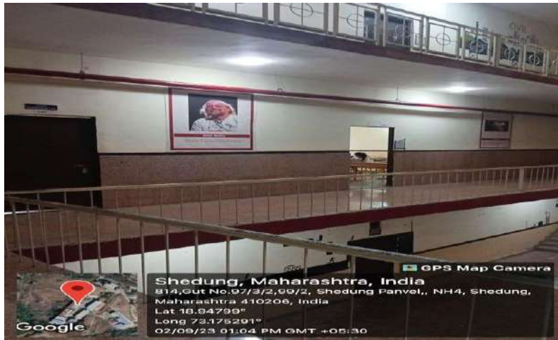
LED Lights in Corridor
